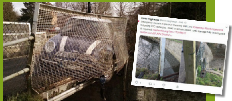
Bridge damage caused by collision, West Essex Road closed until repairs can be arranged
